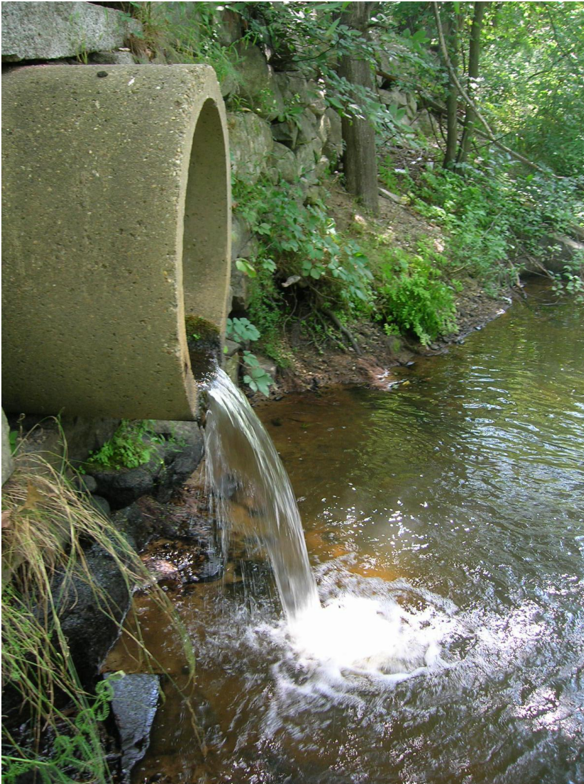
Figure 10: Impassable culvert (perched) on Woodman Brook in the Lower Lamprey River subwatershed.
