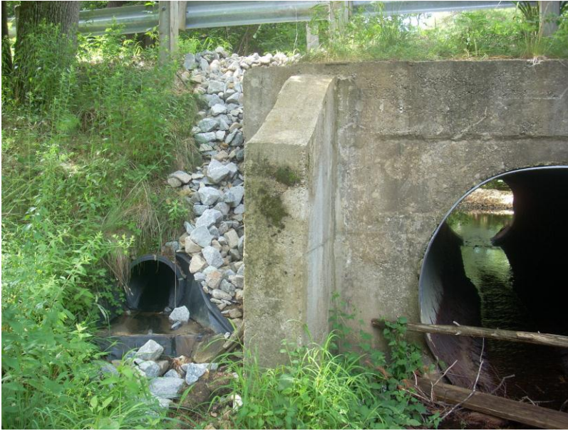
Figure 12: The tail end of a pipe that directs stormwater runoff into Dudley Brook.
