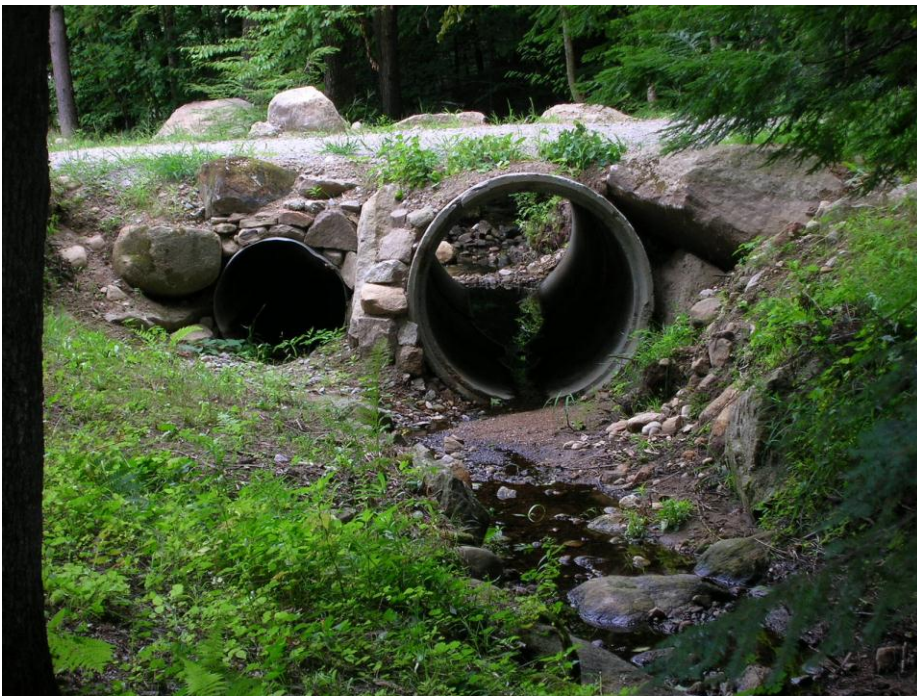
Figure A.20 - This driveway culvert marks the downstream limit of brook trout in Aunt Mary Brook.
