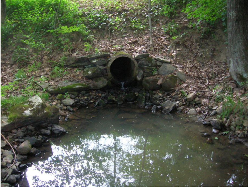
Figure A.24 - Perched culvert above scour pool where brook trout were captured in an unnamed tributary of the lower North River.
