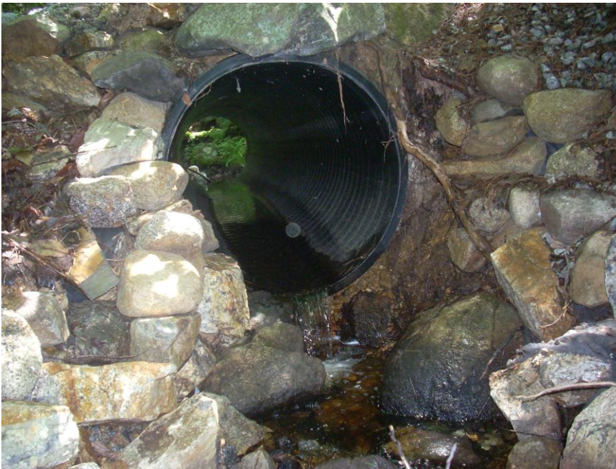
Figure A.6 - One of three driveway culverts impacting fish passage on a coldwater stream in the Lamprey River Headwaters subwatershed.
