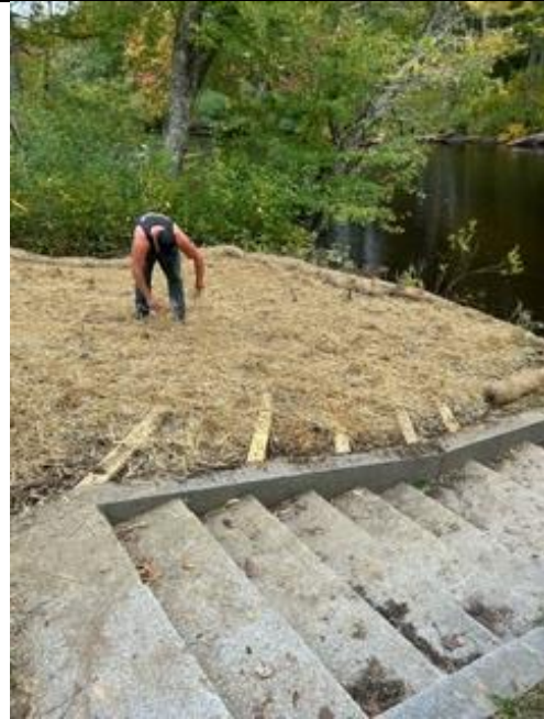
New water bars will help to disperse and divert stormwater, reducing erosion. Once the grass becomes established, paddlers will be able to drag their boats in this area rather than using the stairs.
