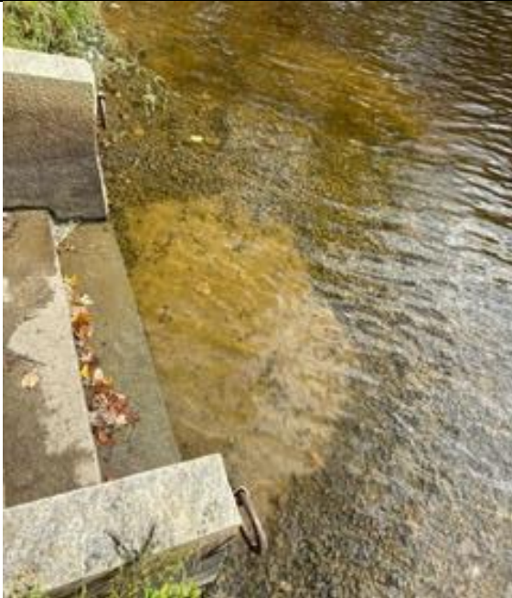
Before the work, the bottom step was being undercut by the river and the step off was a doozy. Now paddlers can step onto a new granite slab without going up to their waists during normal flow.
