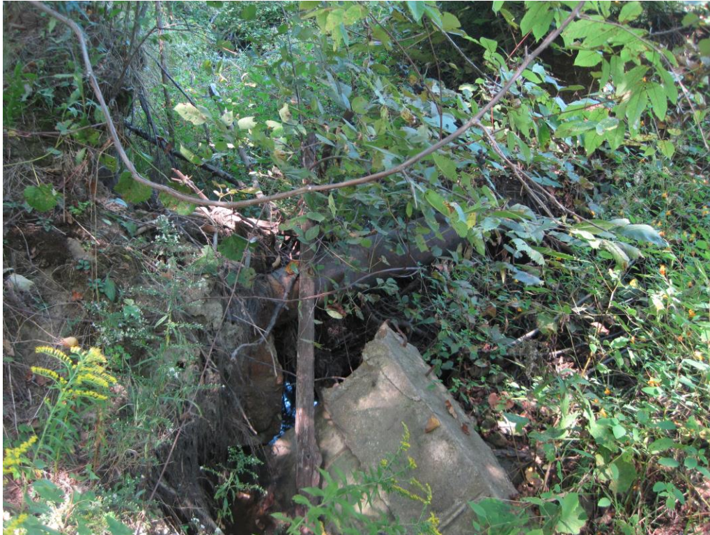
remnants of the discharge pipe
