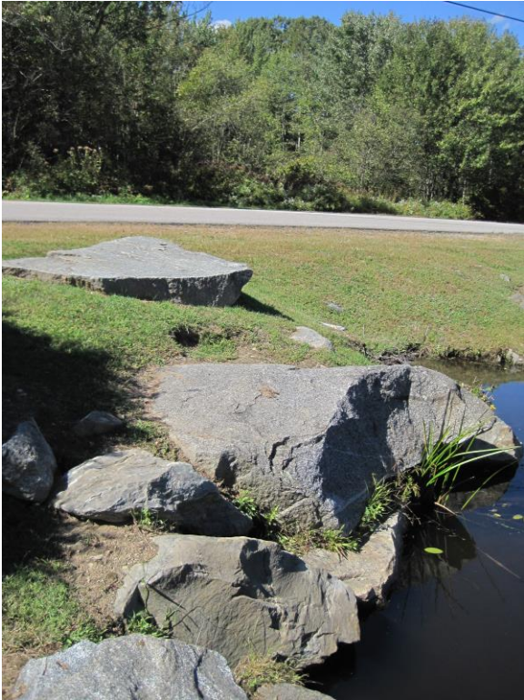
pipe outlet well hidden under these rocks
