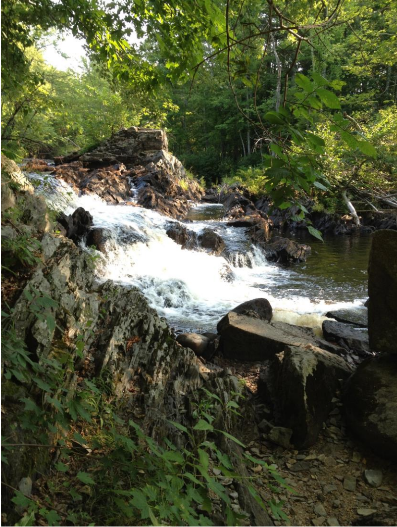
right side of breached dam
