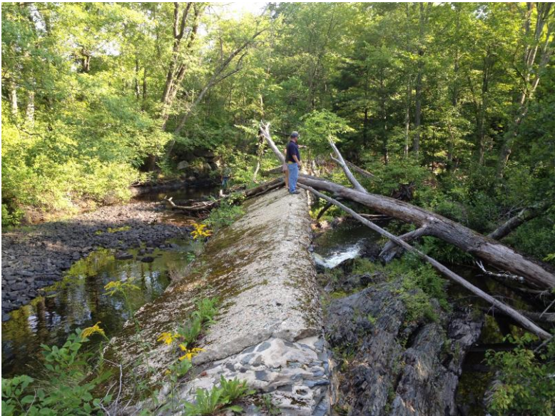
center section of breached dam
