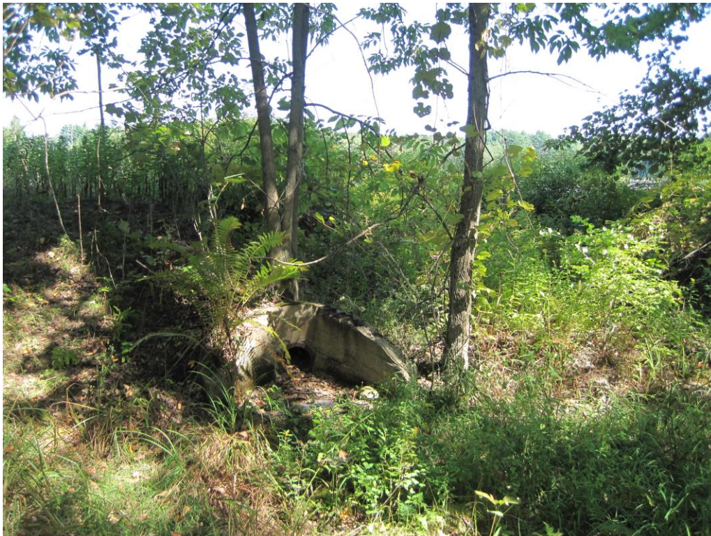
Hoar Pond outlet now by-passed by breached area to right
