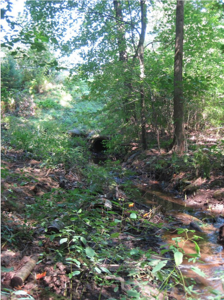
078.05 Melling Glen Woodlands Detention Pond view of dam and outlet and downstream conditions
