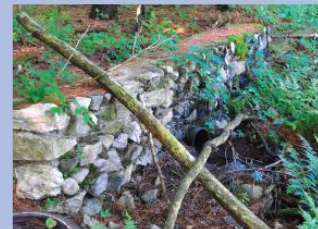
Storm drain pipe emptying into the wetland. Credit: Abigail Gronberg
